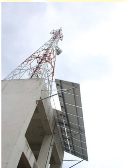
Image 5: Located at Balaganj, Jagannathpur, Sylhet (Innovative GFRT mounted Panel Structure without additional land)
