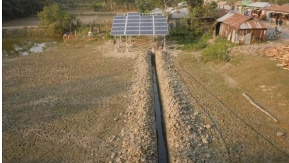
Image 1: Located at Harandra Bazar, Hatiya (40m Underground Cabling from BTS to Solar Panels)
