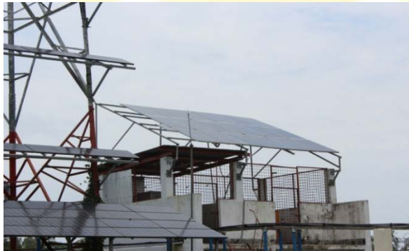
Image 3: Located at Shantiganj Bz, Jagannathpur, Sylhet (Customized Rooftop mounted Solar Panels without additional land)
